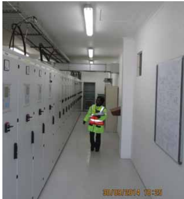
Figure 4-1 : Newly Upgraded Suidwal Substation
