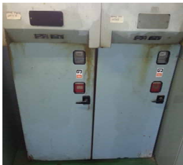
Figure 4-2 : Oil-filled Switchgear at Paradyskloof Substation
